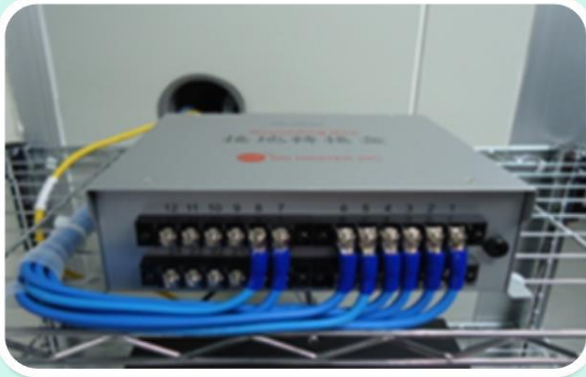
MULTI-GROUNDING SYSTEM MONITOR
